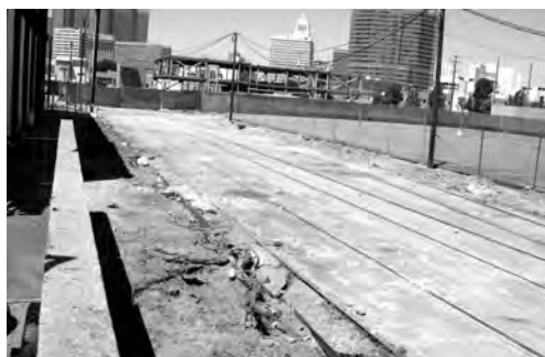
Banning Street, cleared and soon will connect the three sections of the L.A. Betsuin property.
